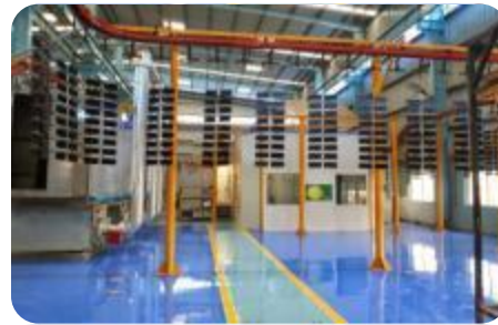
-Powder Coating Plant
