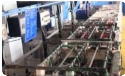
-Nickel Chrome Plating Plant
